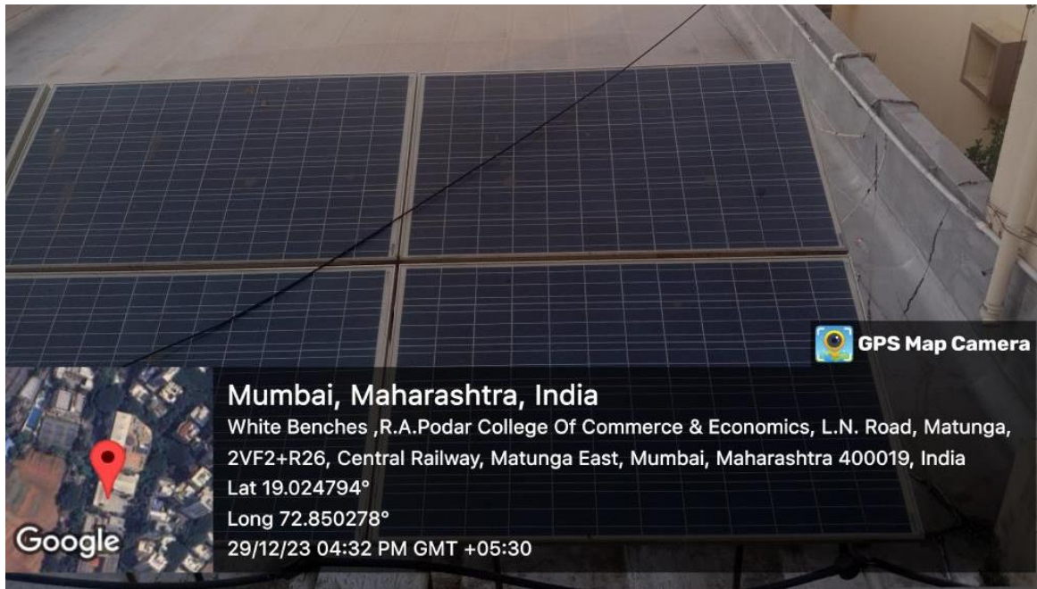
Plate 4: Rooftop solar panels in the terrace area
