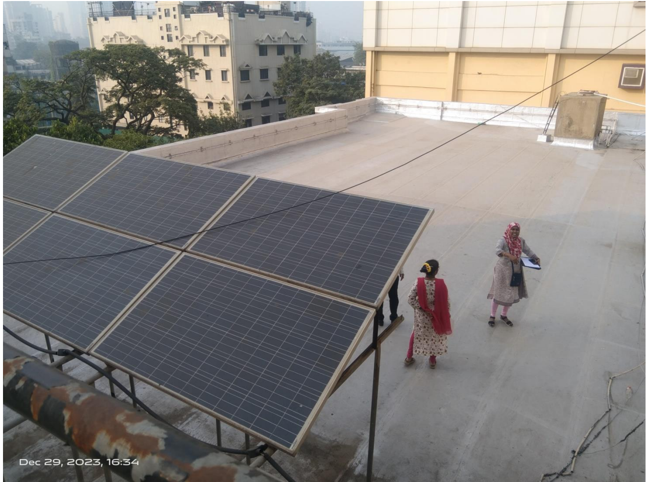
Plate 7: Solar panels on the rooftop
